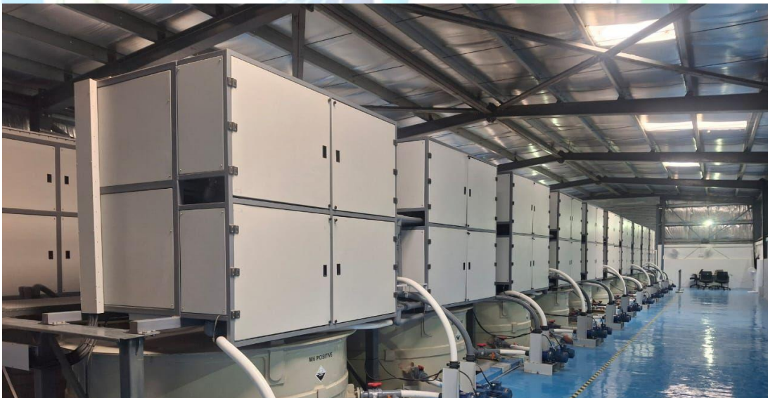
Vanadium Redox Flow Battery Installation
